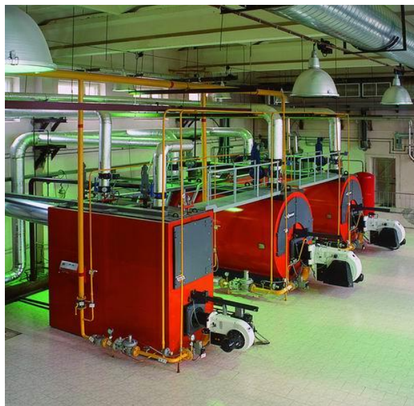
Fig.2. Hot water boilers
