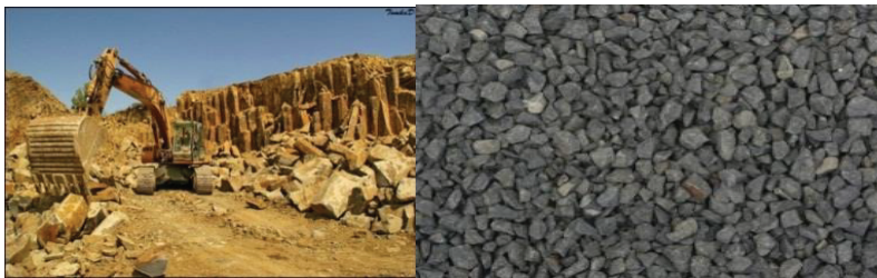
Fig. 1. Extraction and initial stage of processing of basalts from the Aydarkul deposit.
