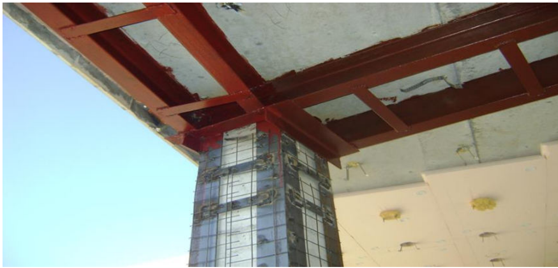
Figure 1. Emergency reinforced concrete column, a state replaced by a unloading system.
